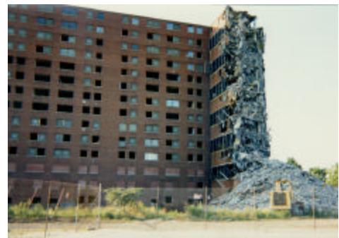
The first stage of the redevelopment of the Henry Horner Homes was the demolition of five high-rise buildings,
